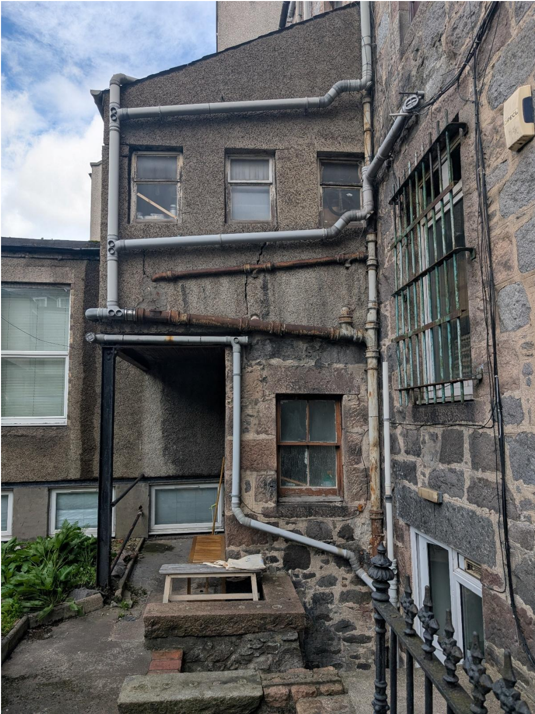
Fig. 1 – Rear washhouse/toilet block showing extensive cracking to harled brickwork and multiple rainwater/soil pipes.
