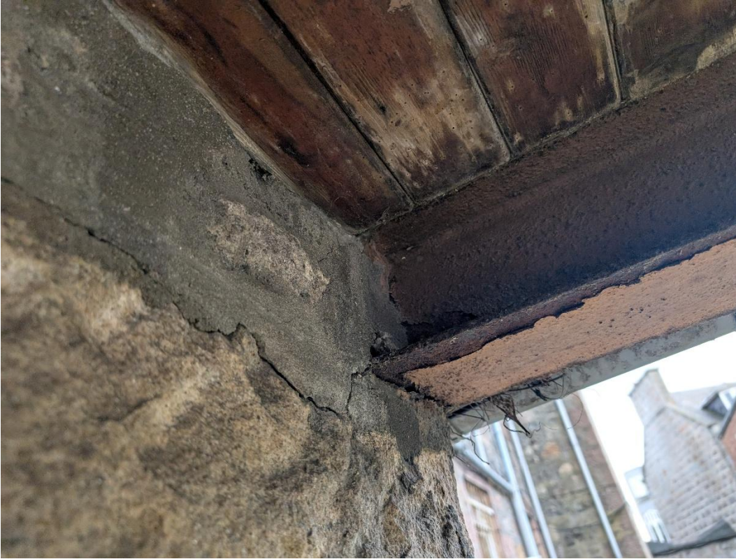
Fig. 2 – Steel beam bearing into masonry with associated cracking.
